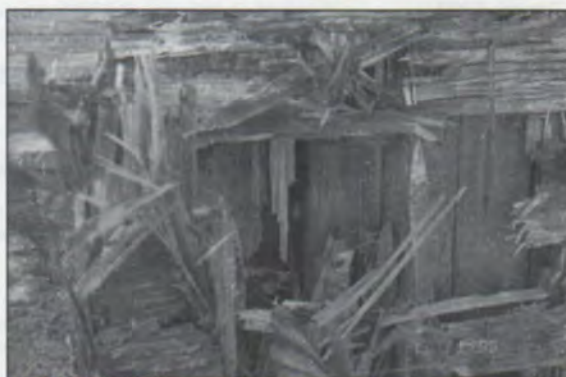
A PCO's nightmare: Wood damage beneath a window in an EIFS building.
