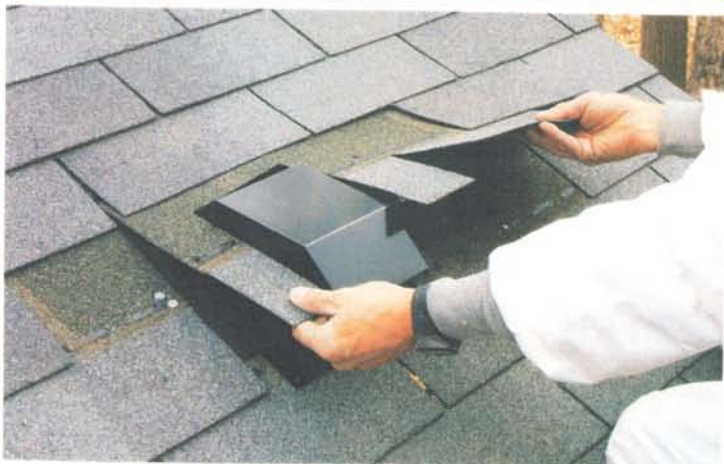
Cut around the vent and replace the shingles. Before the shingles are replaced, they are cut to fit closely around the vent, overlapping the flange on the top and both sides.
