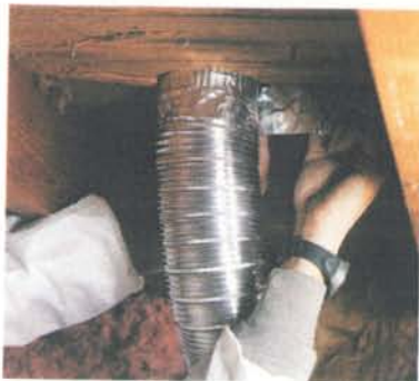
Connect the duct. Back in the attic, the duct is connected to the vent and sealed with aluminum duct tape.
