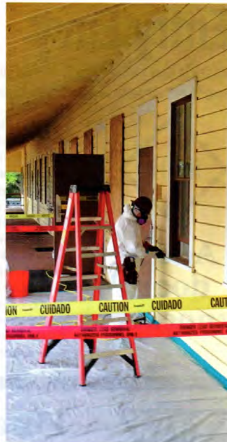
A lead-abatement professional from T. Simons & Co. wears head-to-toe protective clothing and works in a sealed-off area when sanding window sash containing lead paint.
