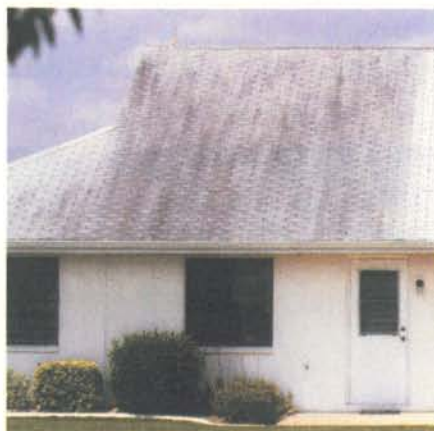
In this test house, the shingles on the left are stained with algae, while the shingles on the right include copper granules from 3M that protect the roof from algae.
