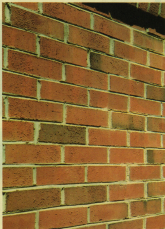
Figure 5. After achieving a mortar match, actually laying the brick is easy. The author is careful to match the pointing technique of the original work.
