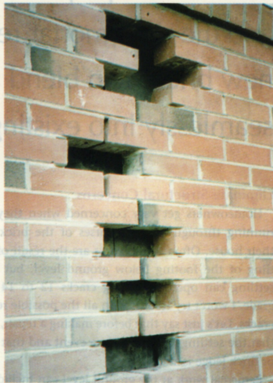
Figure 3. Working slowly, the author removes the cracked bricks without damaging nearby bricks.
