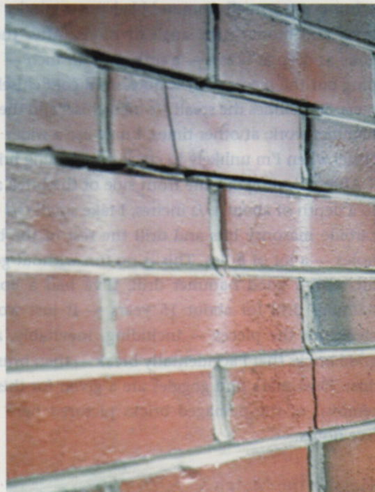
Figure 1. A vertical crack in the brick veneer is often the result of minor settlement in the foundation. Though these cracks typically stop moving and cause no structural problems, most homeowners like them repaired.
