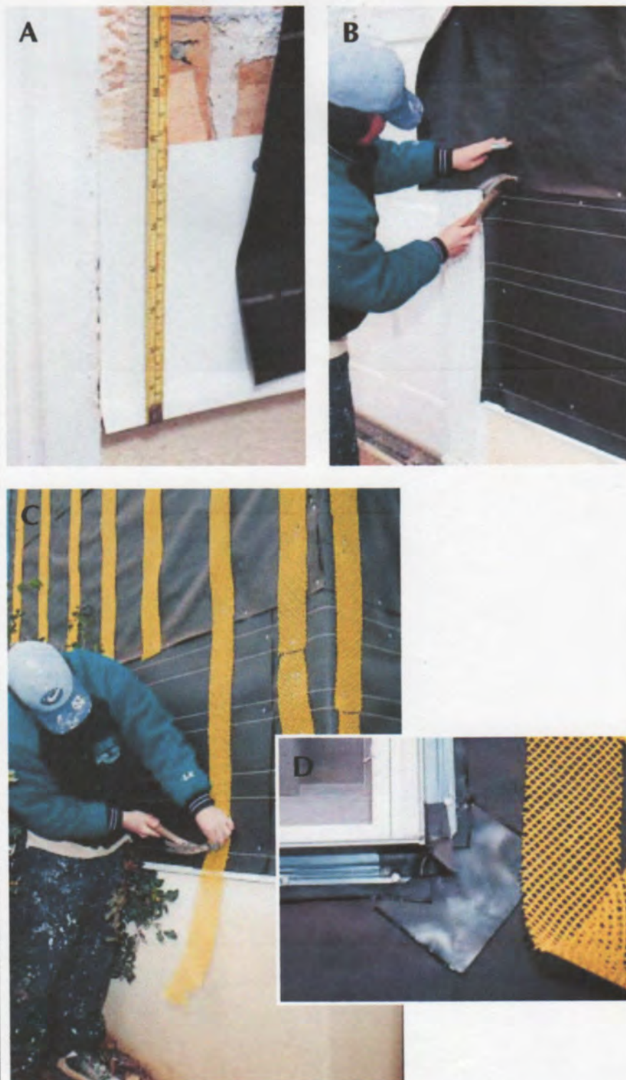
Figure 7. Installation of the drainage plane begins with vinyl or metal base flashing (A). The building is then wrapped in felt paper or Stuccowrap, with 4- to 6-inch overlaps at the joints (B), followed by staple-on mesh furring strips, which provide an air space behind the Durock (C). Extra care is taken to make windows and other openings watertight (D), using a self-sealing barrier tape where needed.
