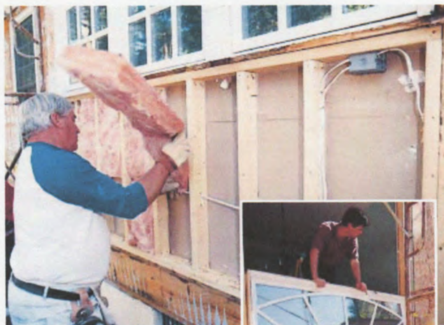
Figure 5. Hidden damage to the structure was discovered during tear-off on the south wall. The wall had to be torn out and replaced, including wiring and insulation (left), and doors and windows (right).
