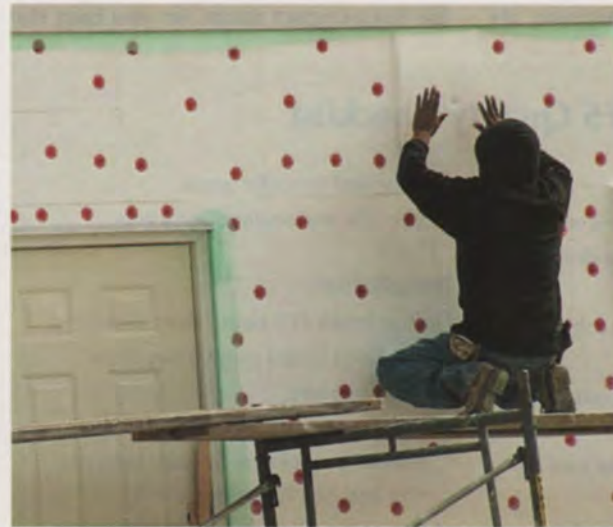
Figure 2. A worker attaches soft EPS "beadboard" with screws to form the base of the EIFS cladding. The close-up, below, shows the voids between the plastic beads. EPS allows water to leak through and can hold moisture against the building. That is why careful joint sealing and an effective secondary weather barrier are critical to system performance.
