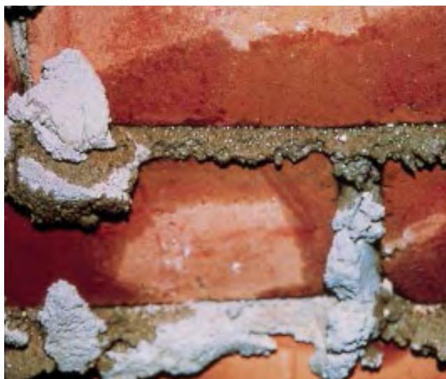
Figure 1. Since wind-driven rain may penetrate brick veneer, it is best to assume that the backs of the bricks will be wet. Unless the water can drain to the exterior, moisture can damage framing or interior finishes.
