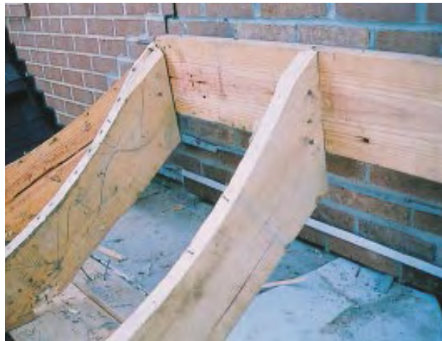
Figure 11. If the flashing at the head of a bay window is placed directly above the lintel (left), it serves no purpose, since it directs water to the interior of the house. The correct location for through-wall flashing above a bay window is above the roof (below).
