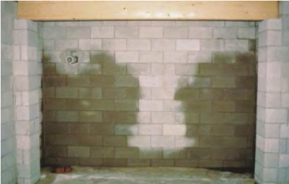
Figure 12. Omitting flashing and weepholes is risky. Water that penetrates brick veneer can saturate wood framing or enter the basement.
