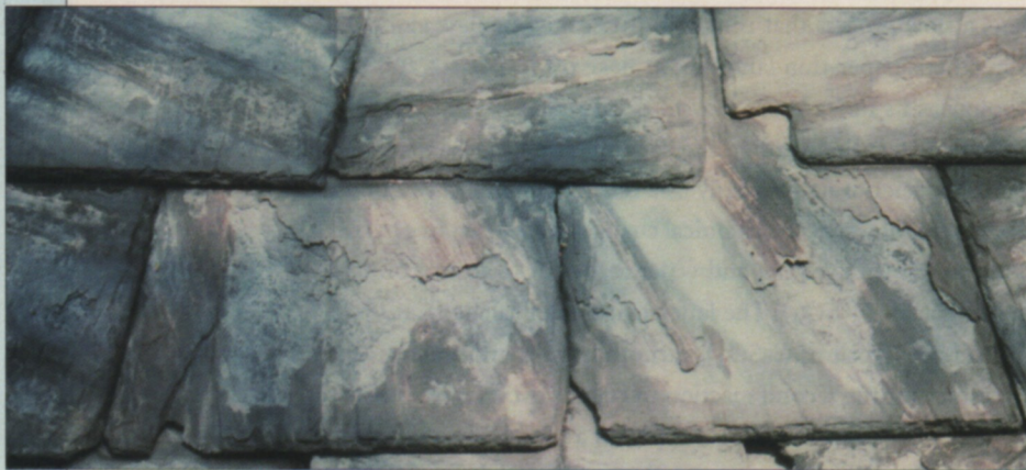
This Pennsylvania Hard-Vein slate has reached the end of its serviceable life. Note the numerous cracks, indicating loss of strength, and the severe delamination that allows the slate to absorb moisture.
