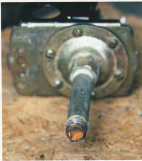
Figure 4. This galvanized pressure switch pipe is completely blocked with corrosion. As a result, the pressure could build to disastrous results or the pump refuse to turn on at all. A brass nipple would have prevented this corrosion.
