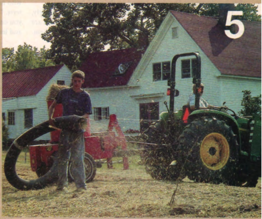
THE NEXT DAY , the contractor backfilled clean sand over the pipes and replaced the topsoil. As a finishing touch, the leach field was seeded with grass and mulched with a layer of hay. With proper care, the system should last 40 to 50 years.
