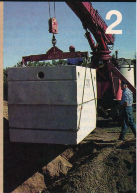
A CRANE OPERATOR lowered in the 3-ton concrete septic tank. After it was set in place and leveled, it was connected to the house with a line of solid sewer pipe. The tank holds 1,250 gallons, enough to support this five-bedroom Maine farmhouse.
