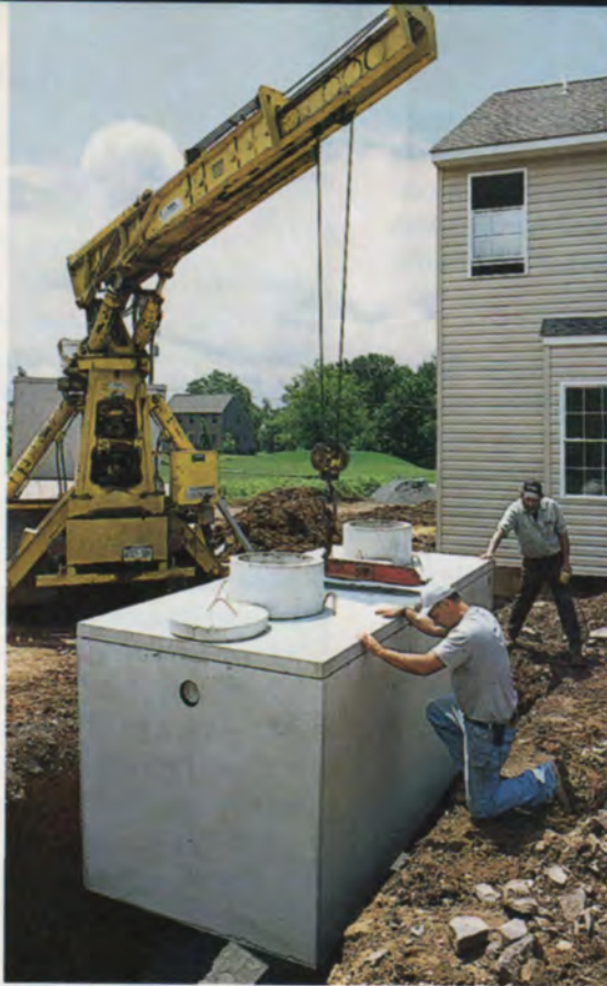
A septic tank is set in place at a new house in Schwenksville, Pennsylvania. The 1,500-gallon tank serves a four-bedroom house and will need pumping every two to three years.
