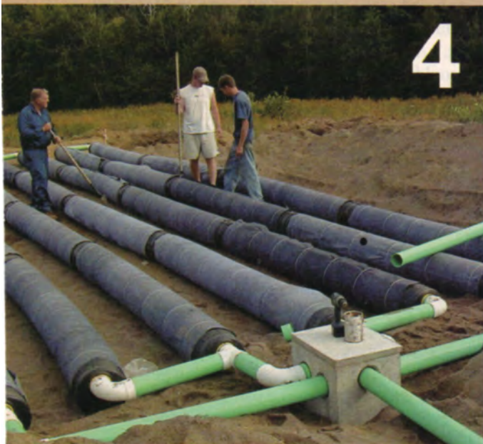
WORKERS LAID OUT and leveled the eight rows of perforated drainpipe. Effluent flows to the leach field through a distribution box that sends the liquid evenly to all pipes, so that none is overloaded. The pipes are wrapped in a geotextile fabric, which keeps out fine sand and aids in the filtration of wastewater.
