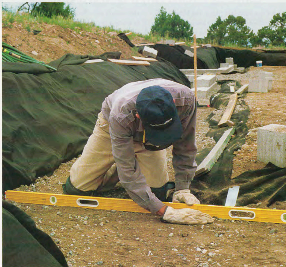
A level start is crucial. Rebar pins driven into the ground on 6-ft. centers act as reference points to level the compacted base material.
