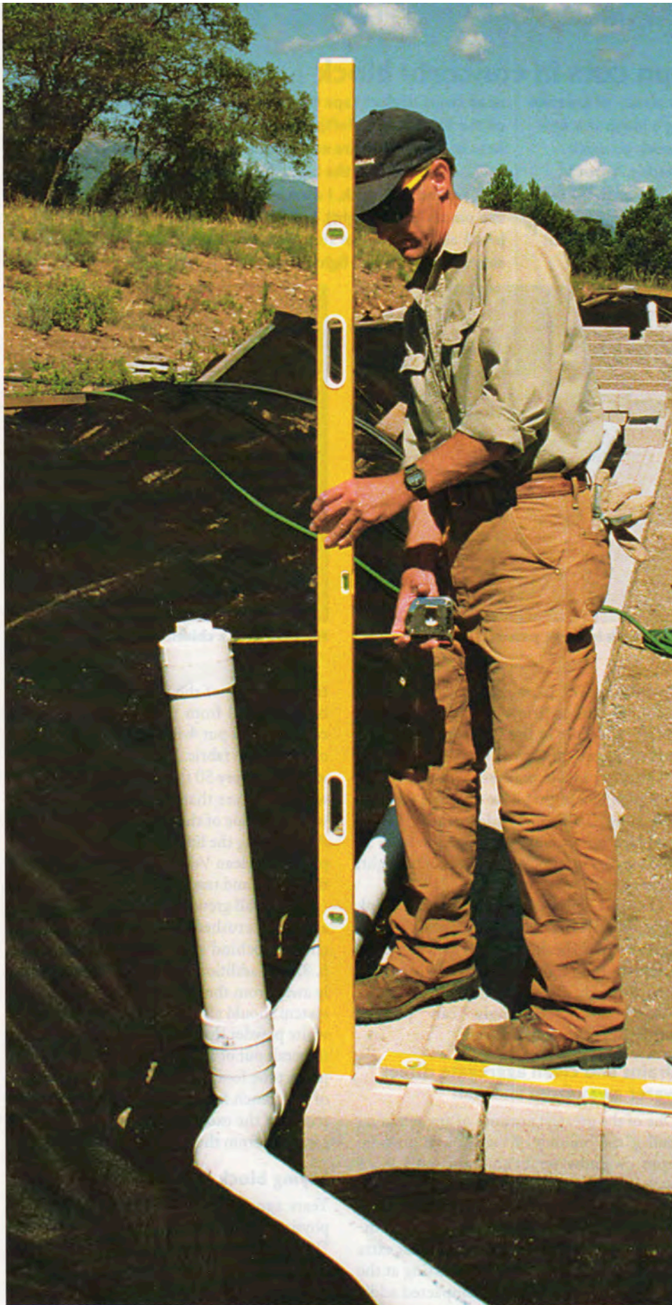
Plumb is not what you want. Clean-out risers for the subsurface drains behind the wall must be pitched back at the same angle as the wall. Over the wall's 4-ft. height, the face tilts back a total of 5¼ in.
