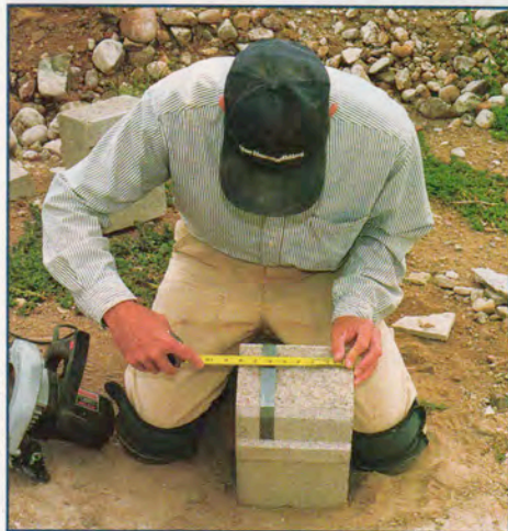
Tape marks the line.
