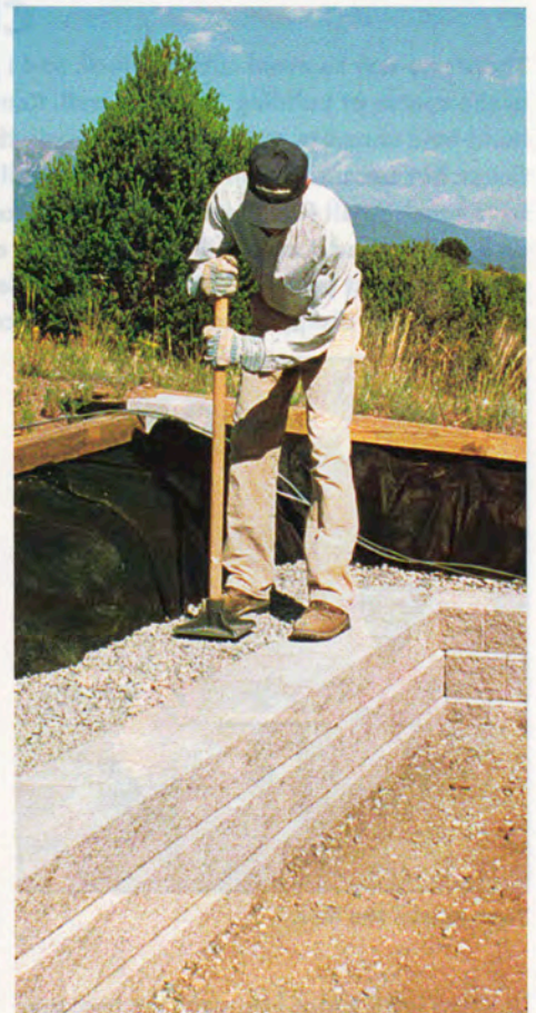
First the block, then the stone. After laying a course of block, the author brings up the level of crushed stone behind the wall and tamps it by hand.
