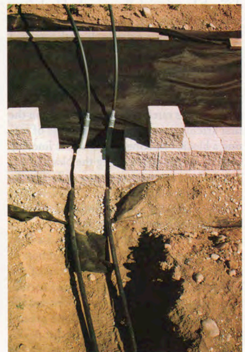
Make way for water. A circular saw with a diamond blade makes the narrow channels for these water lines. Grooves are patched with mortar and buried during final grading.
