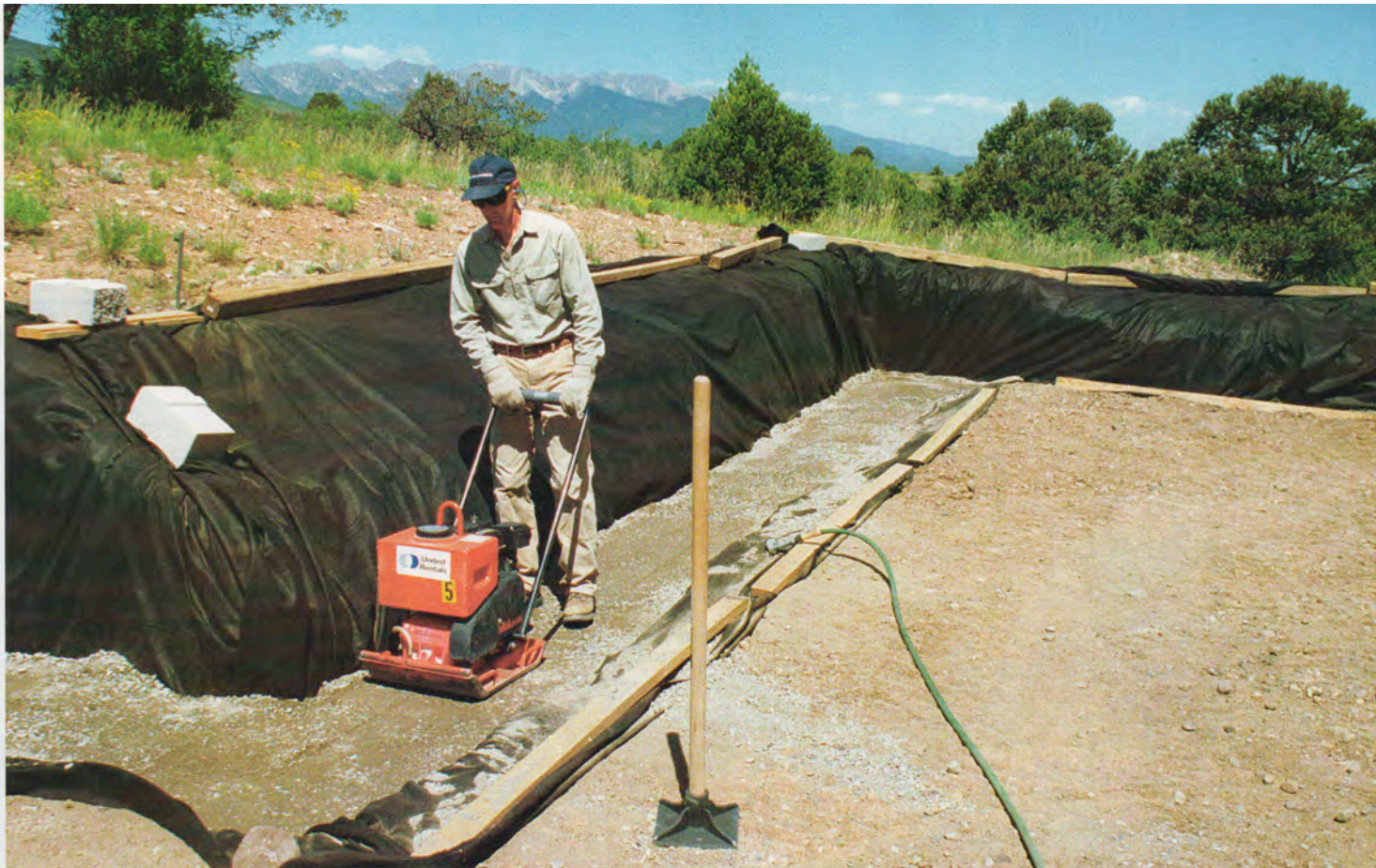
A solid wall needs a solid base. After digging a 12-in. deep trench 30 in. wide, the author compacts a layer of locally available road-base material over a layer of filter fabric to serve as the wall's foundation.
