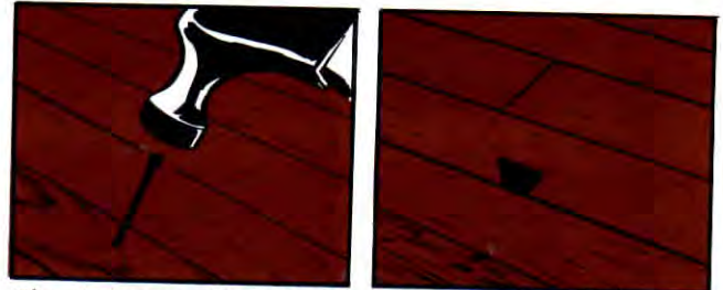
Fig. 3 Face-nailing flooring to remove squeaks and looseness should be at an angle and into a joist or screed. Pre-drilling saves many bent nails.
