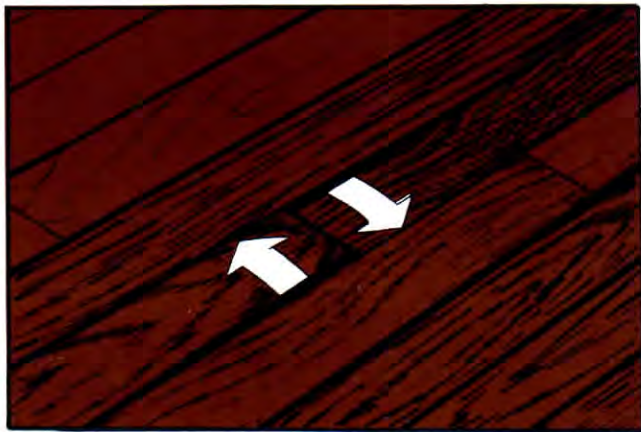
Fig. 5. Cross-pull results when two strips are pulled in opposite directions because of being nailed to different subfloor boards.
