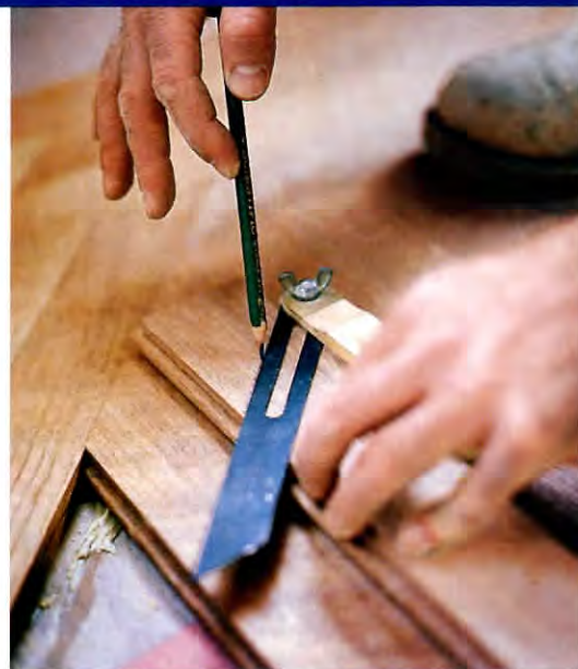
ABOVE: Using a sliding T bevel, Tim Taggart marks the angle of a cut on a strip running the length of the room. BELOW: With a swing of a mallet, his pneumatic stapler simultaneously snugs each strip to its neighbor and anchors the wood to the subfloor.
