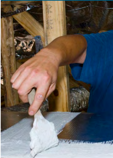
Figure 11.1. Paint mastic (a thick, goeey substance) on to the duct seams and joints. (Photo source: Habitat for Humanity Lakeland FL).
