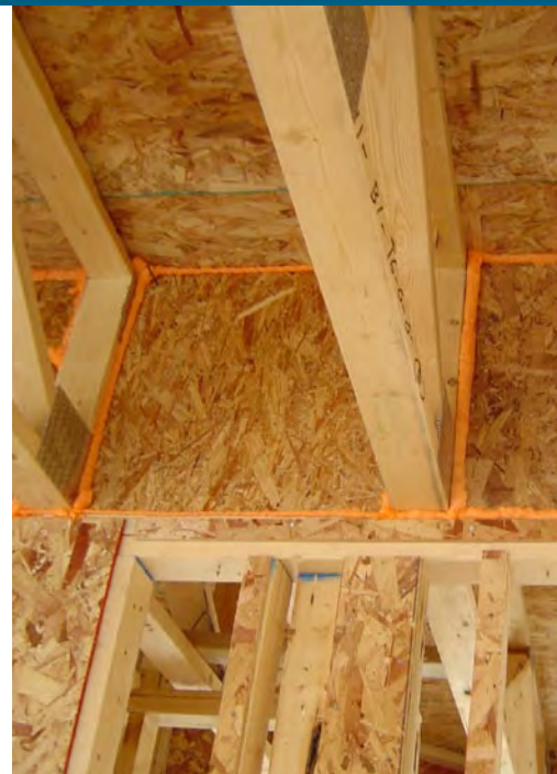
15.2. Seal rim joists of the wall separating the house's living space from the garage with pieces of wall board and spray foam.
