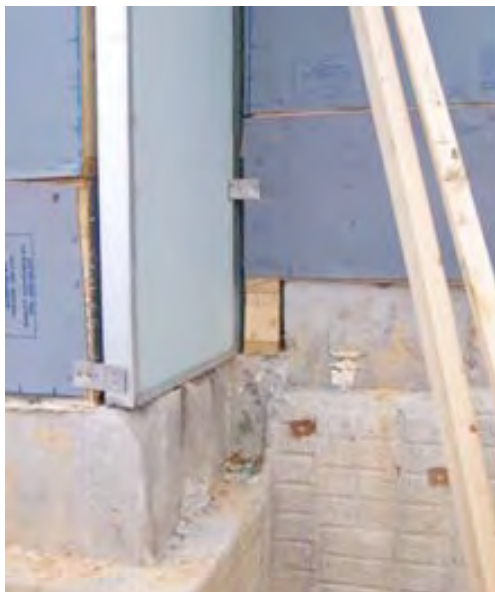
Figure 19.1. Seal air gaps between two framed common walls (Source: Energy Services Group, from EPA 2008)
