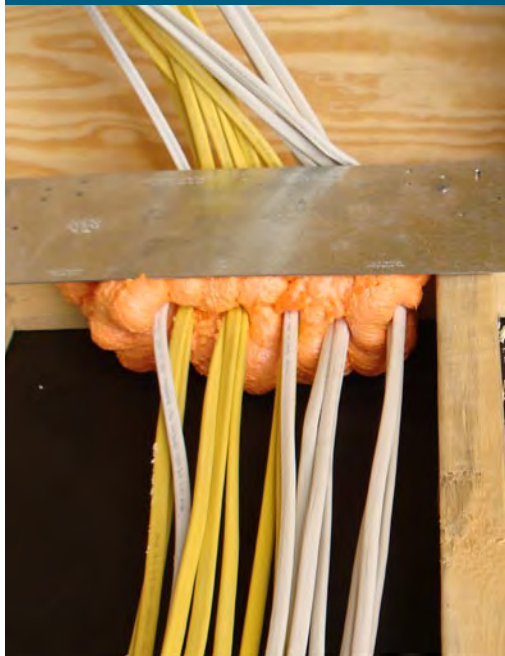
The holes in the sill plate were properly air sealed during construction of this house.
