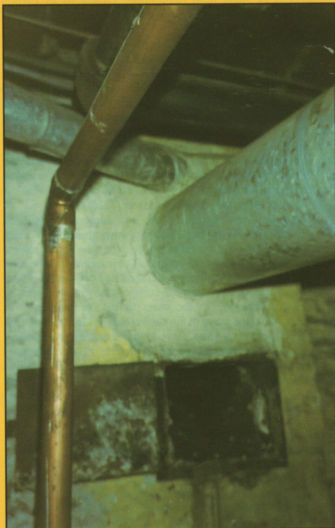
A view of a vent from a recently installed gas-fired furnace with the pre-existing cleanout open and soot and debris visible in the base of the chimney. (Photo courtesy of the City of Albany Building Dept.)
