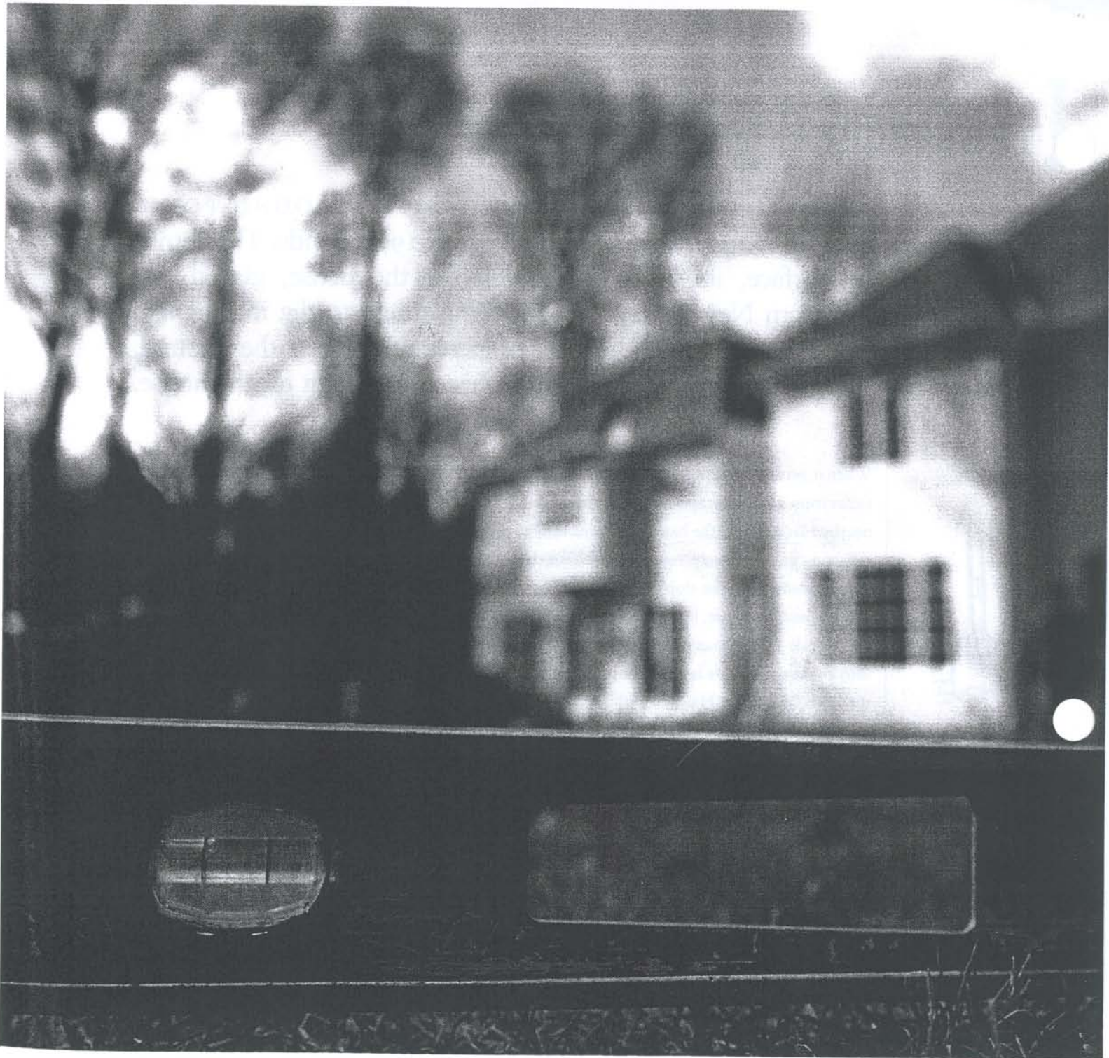
The bubble in the level signals part of the problem: a slope that sends storm runoff and snowmelt toward the house, where it not only floods flatter ground but also pours into the basement.
