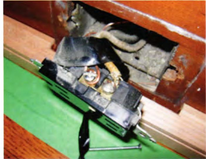
Old wire can easily be identified with the removal of cover plates; however, we don't recommend pulling the outlet out of the box.
