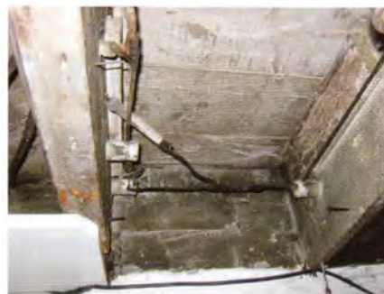
Although these circuits are obsolete, the original connections that were made with the dull black cloth were correct.
