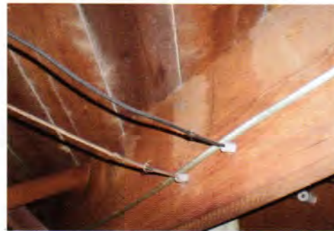
Ceramic tubes can be seen going through the joists and the knobs can be seen in the background. The hot and neutral wire have been damaged.
