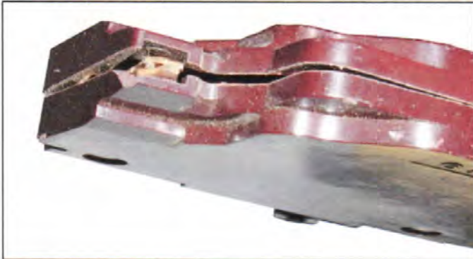
Fig. 7 - Receded Stab in Single-pole E Breaker
