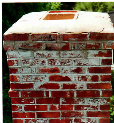
Figure 3. Flue liners should project at least 3 inches above the crown. Here, a thin crown and recessed flue liners caused this chimney crown to leak. As the water worked its way out of the chimney and evaporated, soluble salts remained behind, leaving a whitish stain called efflorescence.
