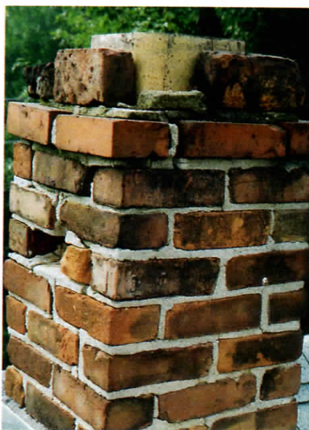
Figure 8. Older chimneys with deteriorated lime-and-sand mortar must be torn down to the roofline and rebuilt.
