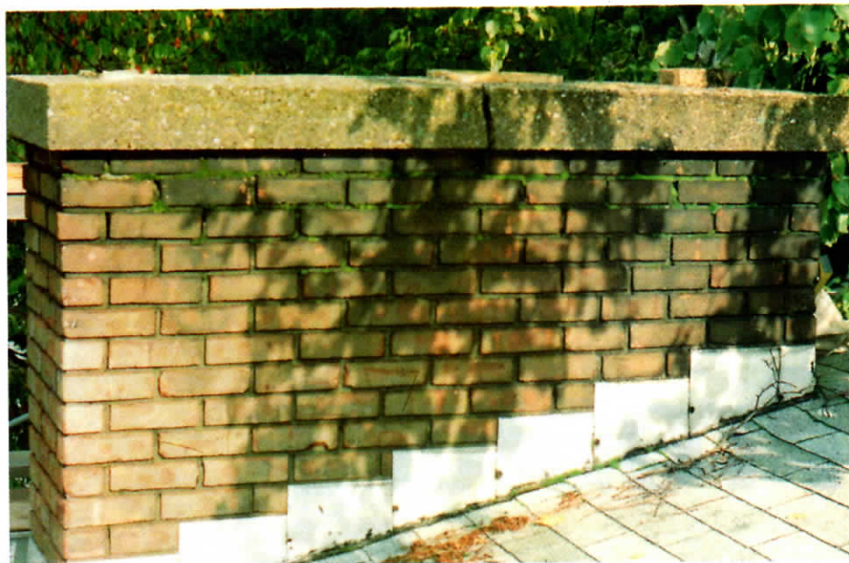
Figure 2. Excessive shrinking caused this crown to crack at the weakest point — the area where a flue penetrated the surface. Proper curing reduces the amount of shrinkage, and reinforcing fibers added to the concrete crown mix add tensile strength.
