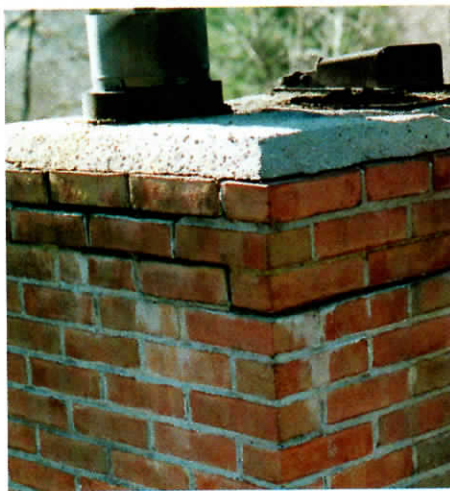
Figure 1. This chimney crown dried too quickly, causing the edges to curl and pull away from the masonry, allowing water to penetrate. This crown also bonded to the flue liners. When the liners expanded, they lifted the top of the chimney, causing the top three courses of brick to crack.
