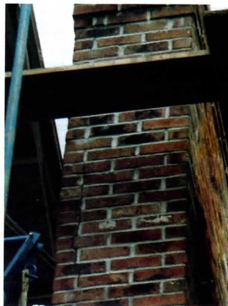
Figure 5. The code-required air space between the flue liners and the chimney walls allows the liners to expand and contract freely. In this chimney, the void between the bricks and the flue liners was filled solid with mortar, and resulted in a 7-foot-long crack when the liners expanded.
