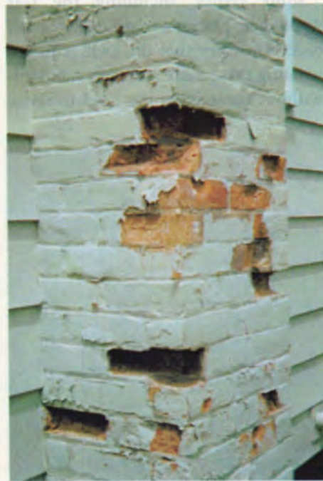
Masonry chimneys can be damaged when corrosive flue gases condense in cold, oversized flues. Exterior chimneys like this one are particularly subject to condensation.
